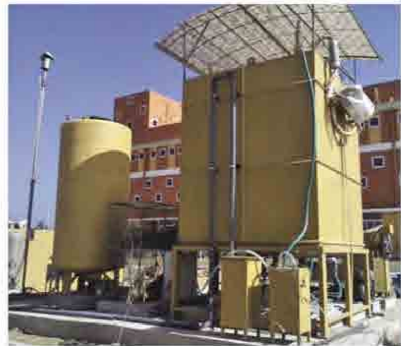
» GPS's BioUrja (Bio waste to energy digester) at one of the largest University Campuses
